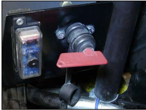
Fig. 8-7 Switching on the power
